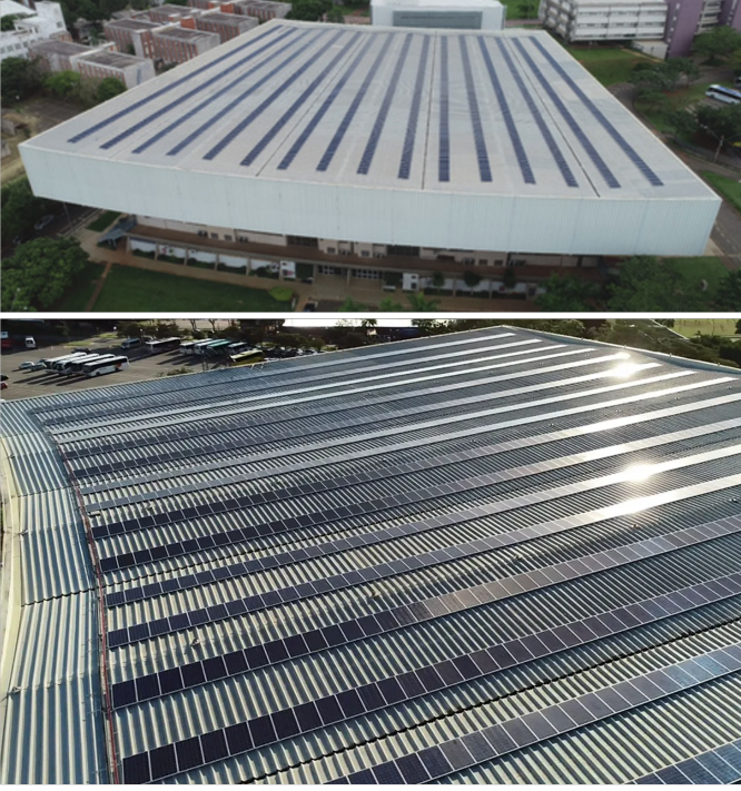
Fig. 2. PV plant installed at UNICAMP [26].
